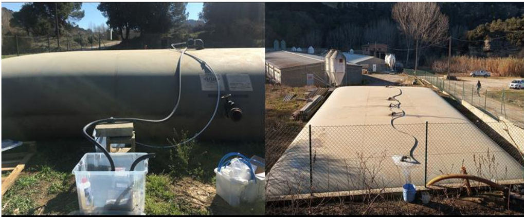
Storage system for biogas production
