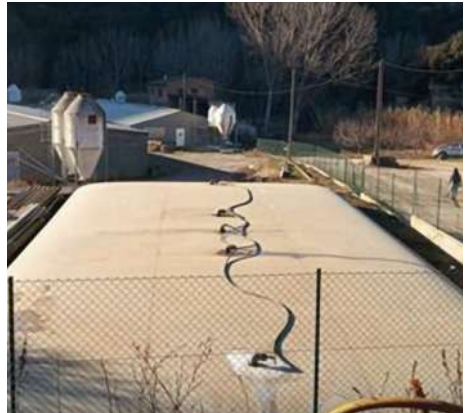
Biogas production – stored slurry covered and methane collected
